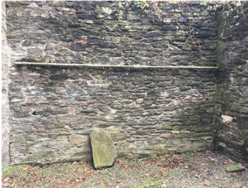
Photo 8.3.1: Surface mounted pipework (possibly gas) leaving the Guildhall (on the left) and heading towards the cottages (on the right)
