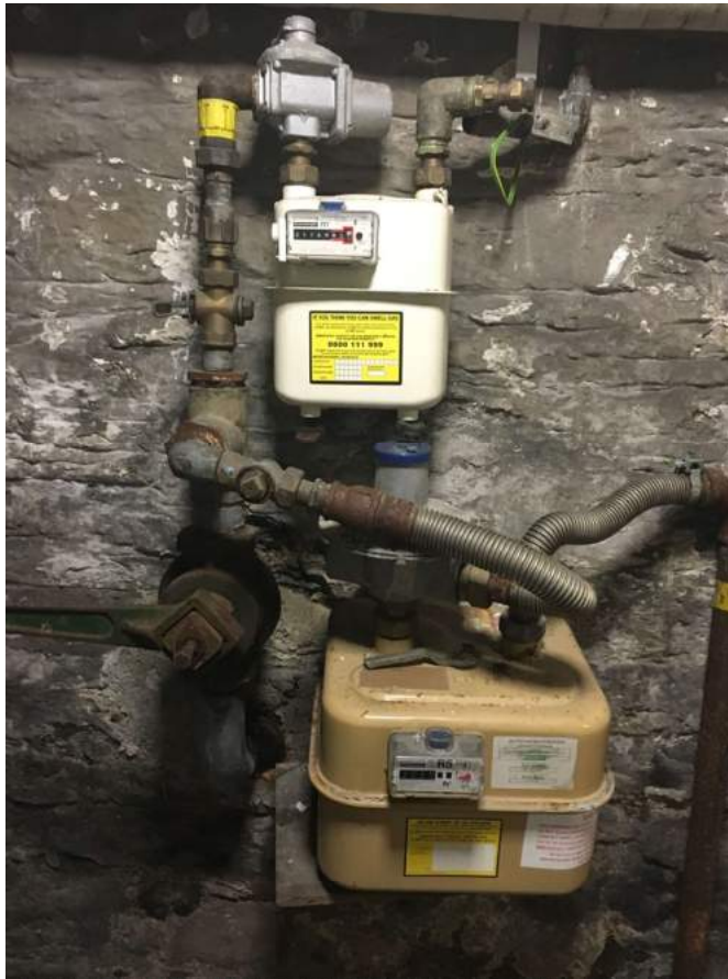
Photo 8.2.2: Existing gas meter(s) (U6 at H/L and U16 at L/L) located in one of the original cells
