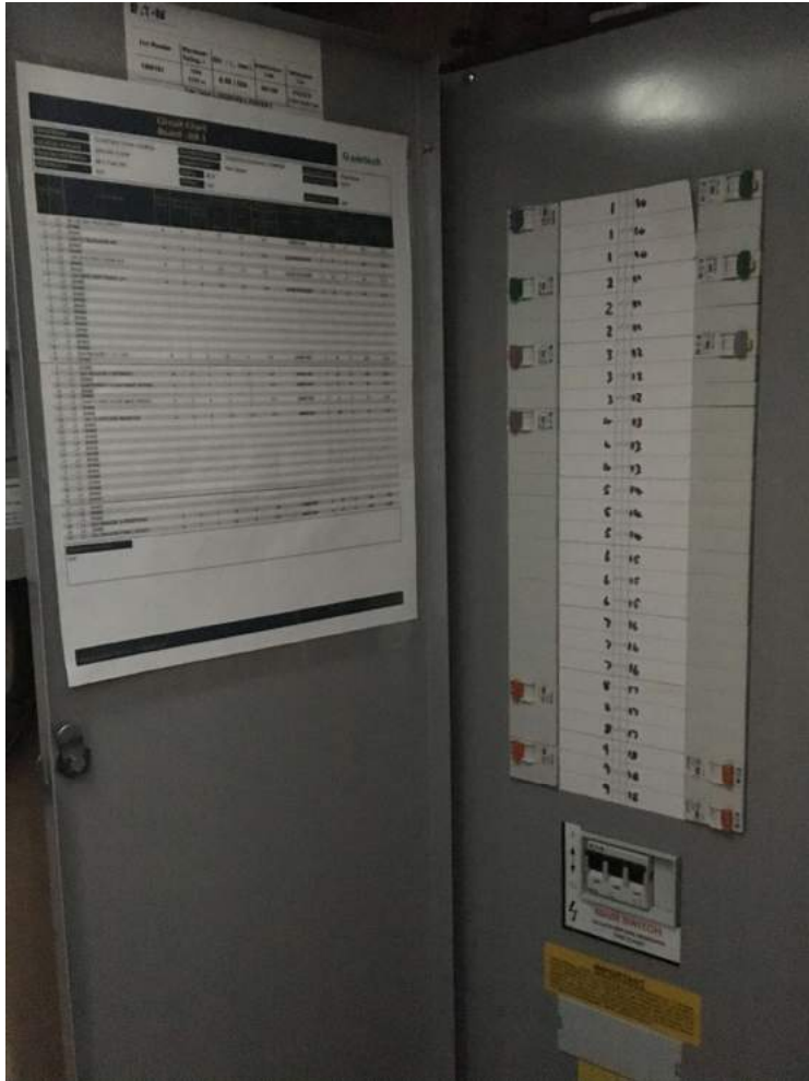
Photo 13.3.1: Recently up-graded panelboard (will be retained)
