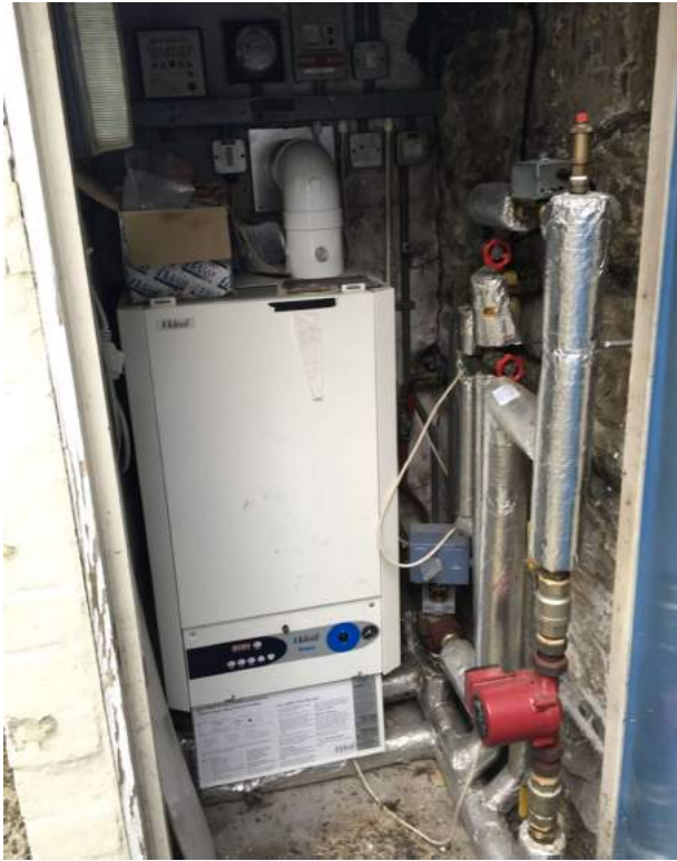
Photo 10.2.1: Existing boiler in lean-to boiler house (will be stripped-out)
