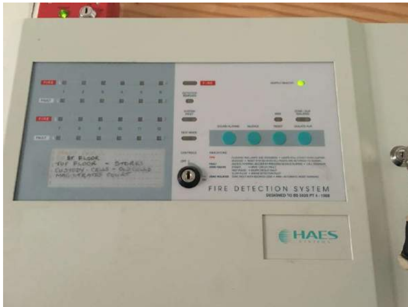
Photo 22.2.1: Existing fire alarm panel at high level (above doorway)
